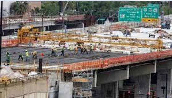
I-4 Ultimate Project - Design Build team for Fiber Optic Network and ITS Devices $9,000,000
