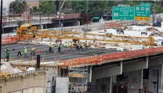
I-4 Ultimate Project - Design Build team for Fiber Optic Network and ITS Devices $9,000,000
